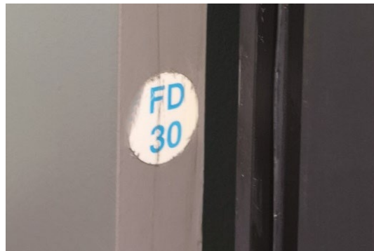
Fire door resistance rating signage
